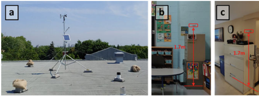
Fig. 259.1 Installations of the, a weather stations and b, c indoor sensors in buildings
