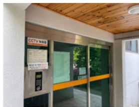
Common entrance control system
