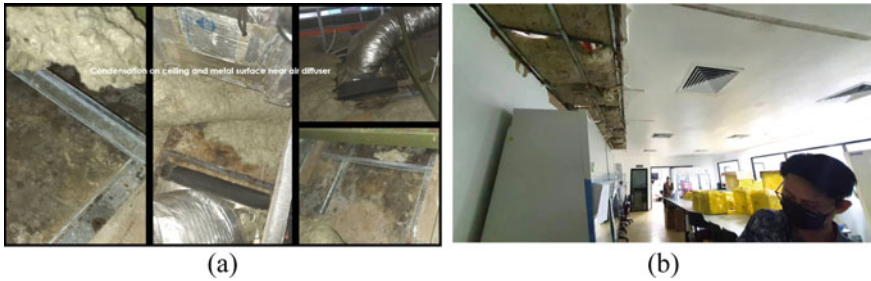
Fig. 2 Incident of ceiling cave in due to heavy condensation build up above ceiling
