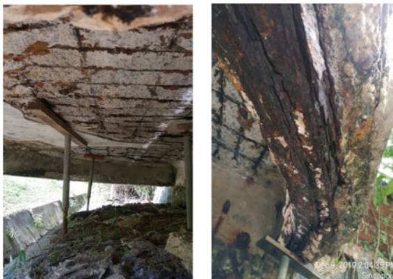
Fig. 2 Severe corrosion in steel reinforcement bars of slabs and beams
