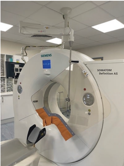
Fig. 8 Photograph of interventional CT set-up with ceiling-mounted protective lead screen. Image Courtesy of Tallaght University Hospital, Dublin
