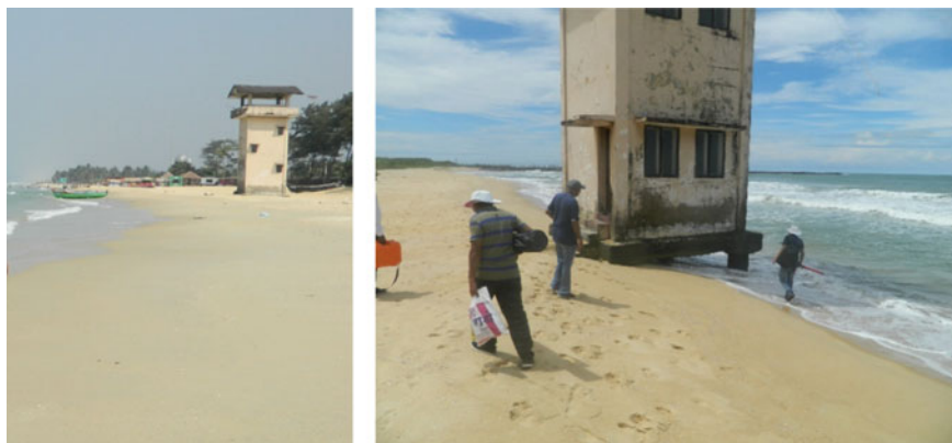
Fig. 8 Comparison of erosion near security post in February 2020 and September 2020
