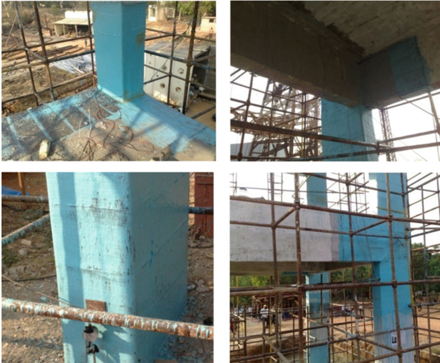
Fig. 10 Structural elements, components and system after retrofitting with FRP techniques and micro concreting
