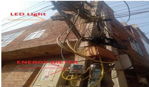
Fig. 1 Streetlight LED and electric meter in Harsh Vihar, New Delhi
