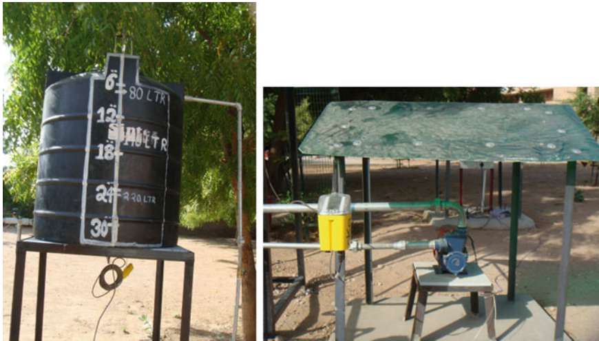
a. Water Tank
