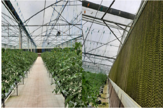
Fig. 6.3 Smart greenhouse with cooling pad system at Nudira Farm, West Java
