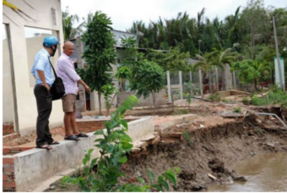
Fig. 3 Housing was eroded in Nhon Duc Ward, Nha Be District (Authors, 2019)
