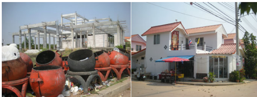
Fig. 4 (Left) the under-construction community center at BEA Ban Ped community, Khon Kaen Province and (right) house modification of BEA at Ban Ped Community. Source Author, 2017
