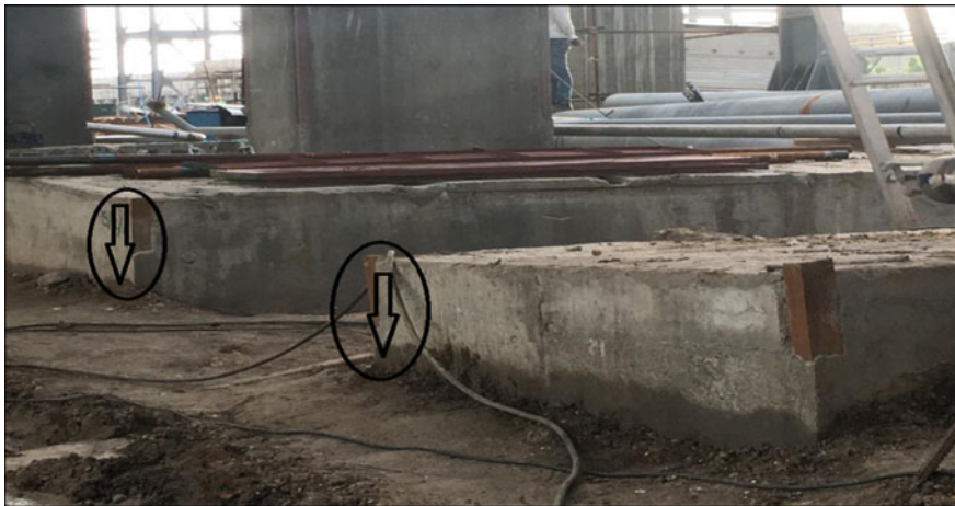
Fig. 5 Differential settlement of pump foundations under self-weight
