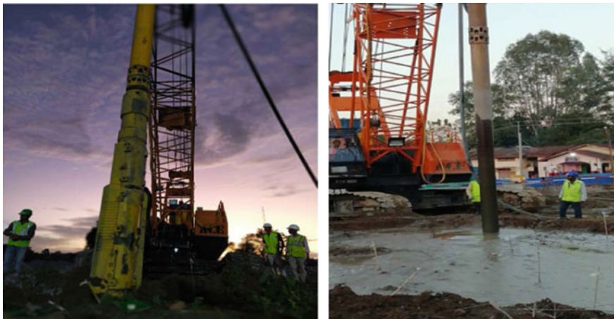
Fig. 4 Typical crane setup by Wet Top Feed Method at Tezpur site (Courtesy: Keller)
