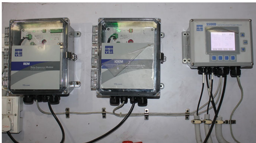
Fig. 11.10 Real-time DO monitor and alarming system (YSI 55000D) used at ICAR-DCFR, RAS facility at Bhimtal
