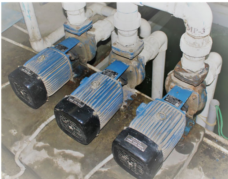
Fig. 11.9 Multiple centrifugal pumps used in RAS facility at ICAR-DCFR, Bhimtal
