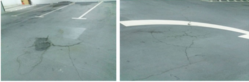
Fig. 5.8 Punching shear cracks in the raft
