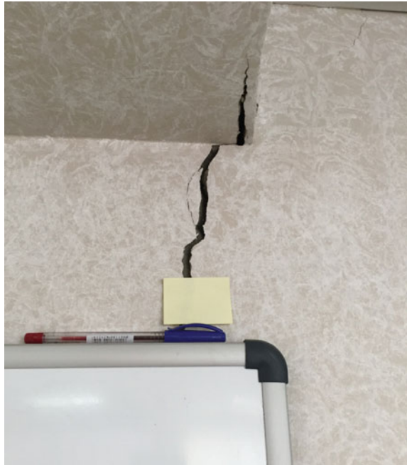
Fig. 2.44 Cracks at the edge column
