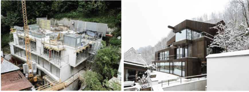
Figs. 2 ALN offices & residential housing by ALN architects, building process and finalized ( Photo Author, Gabriela Obert )
