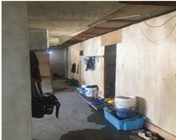
Fig. 2 Construction site A makeshift workers' quarters' set-up made of plywood partition boards
