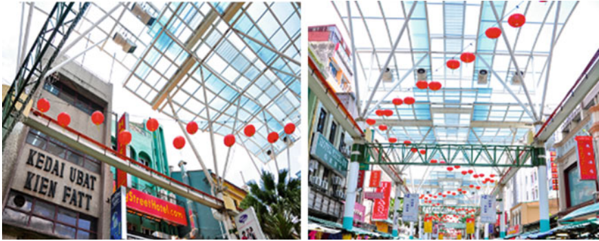
Fig. 3 Huge gaps between roof and building
