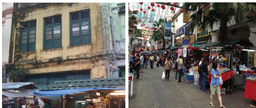
Fig. 5 Dilapidated shophouse and Kiosks arrangement
