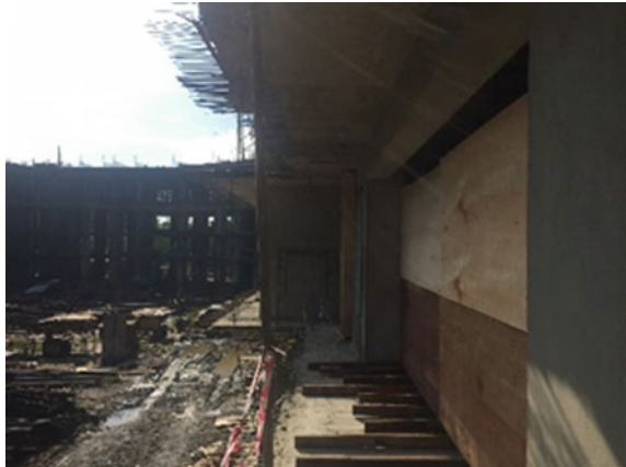
Fig. 1 Construction site A makeshift workers' quarters' set-up within a building undergoing construction
