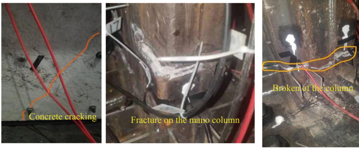
(a) Deformation and damage of the BRSW-1
