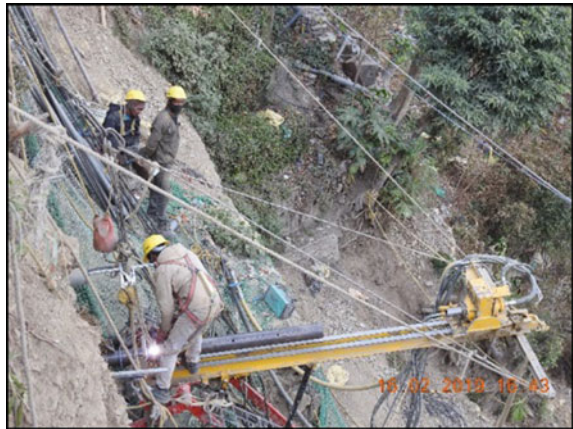
Fig. 11.10 Drilling and installation of soil nail by top-down method at existing valley slope “Tindharia I”. Courtesy M/s. Reinforced Earth India Pvt. Ltd
