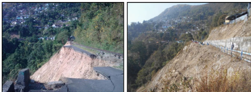
Fig. 11.3 Conditions of landslide affected valley slope at “Tindharia II”
