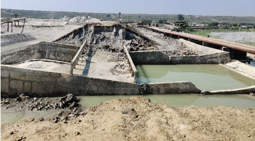
Fig. 41.3 Breached dyke view from top
