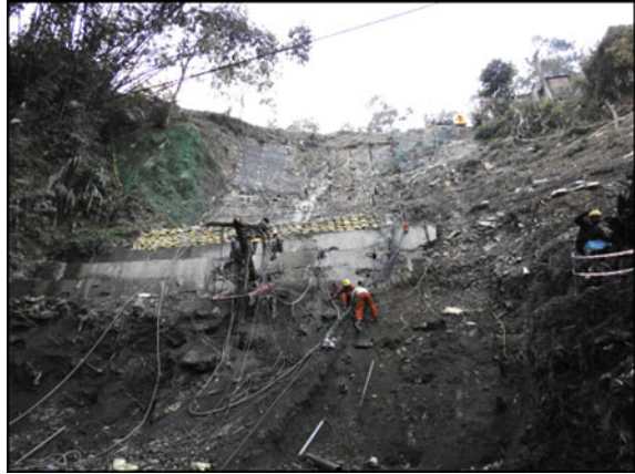
Fig. 11.9 Activity of surface cleaning, drilling, and fixing of welded wire back mesh simultaneously with soil nailing of existing valley slope at “Tindharia I”. Courtesy M/s. Reinforced Earth India Pvt. Ltd
