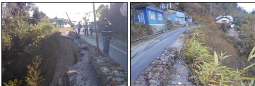
Fig. 11.2 Conditions of landslide affected valley slope at “Tindharia I”
