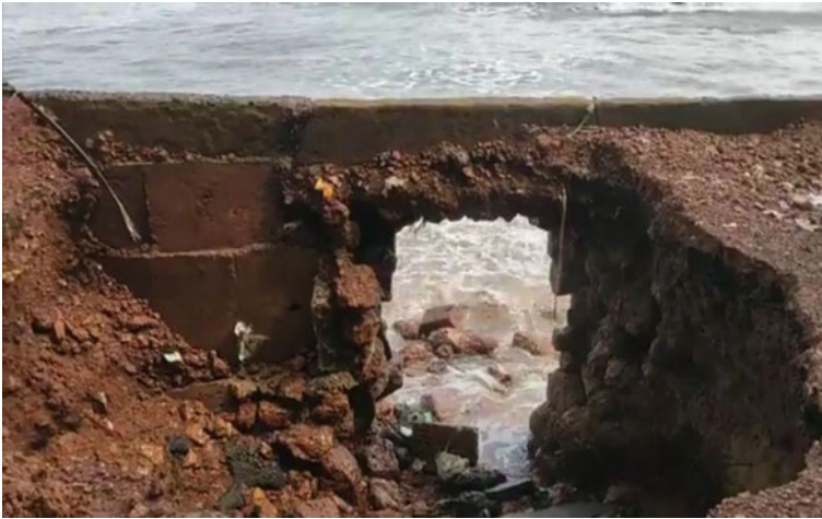
Fig. 36.3 A view of breached retaining wall
