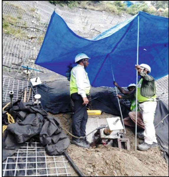
Fig. 11.11 Pull-out test on the steel nailing of existing valley slope. Courtesy M/s. Reinforced Earth India Pvt. Ltd
