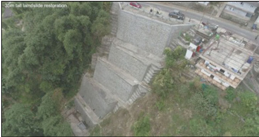
Fig. 11.13 Completed restoration work for valley slope at “Tindharia I” on NH55 (Courtesy: M/s. Reinforced Earth India Pvt. Ltd)
