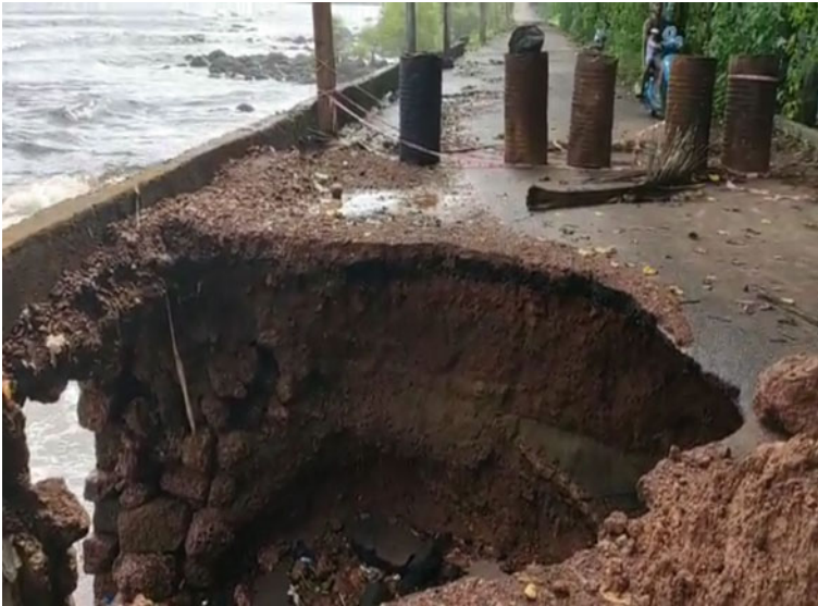
Fig. 36.2 A view of the road caved in
