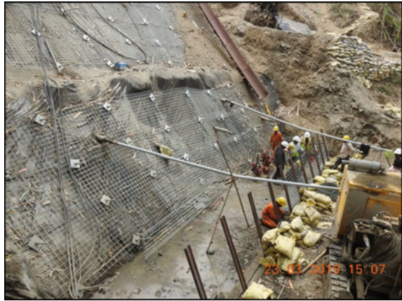
Fig. 11.12 Base level of TerraLink® structure before start of filling and compaction. Courtesy M/s. Reinforced Earth India Pvt. Ltd
