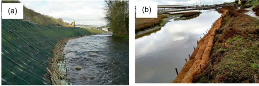
Fig. 2.19 Stabilization of river bank using (a) Turf reinforcement matrix (b) Coir logs (Aditi 2020)
