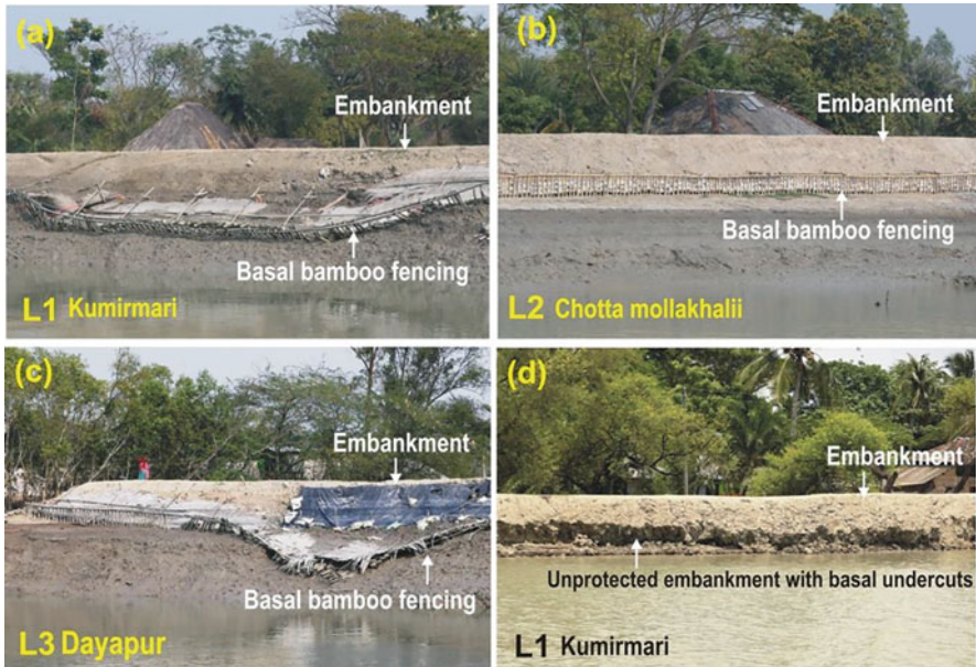
Fig. 7.3 (a–d) Photographs of the embankments the surveyed locations, with protective basal bamboo fencing (a) L1—Kumirmari, (b) L2—Chotta Mollakhali; (c) L3—Dayapur; (d) portion of unprotected embankment with the formation of basal undercuts at location L1
