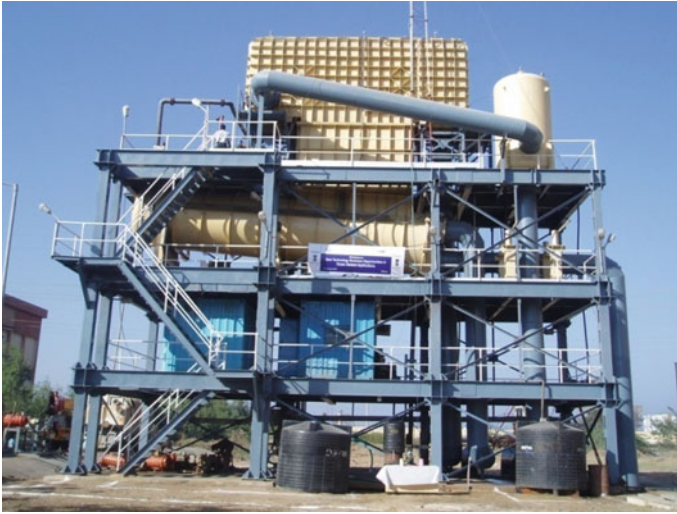
Fig. 12 NCTPS desalination Plant
