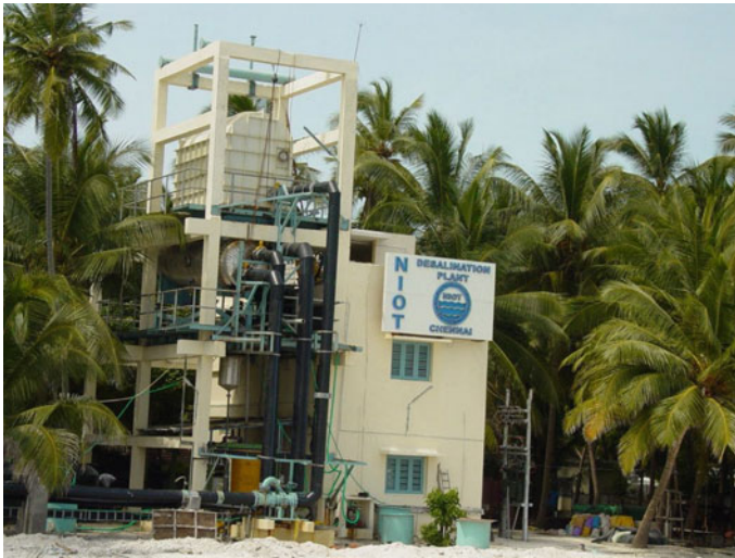
Fig. 7 Desalination Plant at Kavaratti
