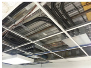
(a) Sensors in Ceiling
