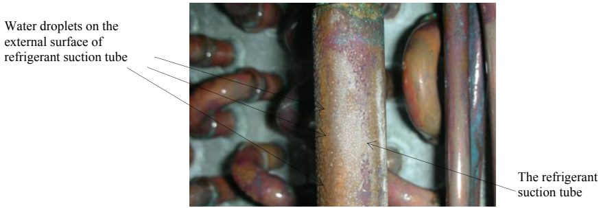
Fig. 4.8 Water droplets formed on the surface of a refrigerant suction pipe
