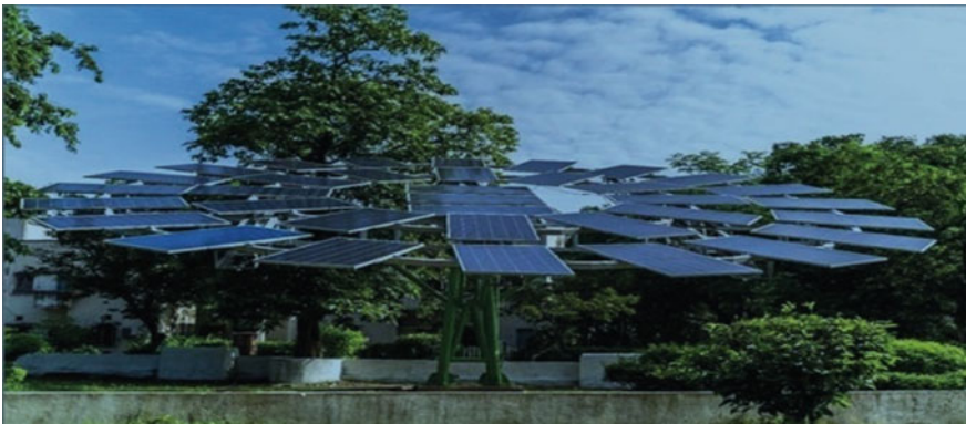
Fig. 6 11.5 KWp solar tree at CSIR-CMERI, Durgapur [17]
