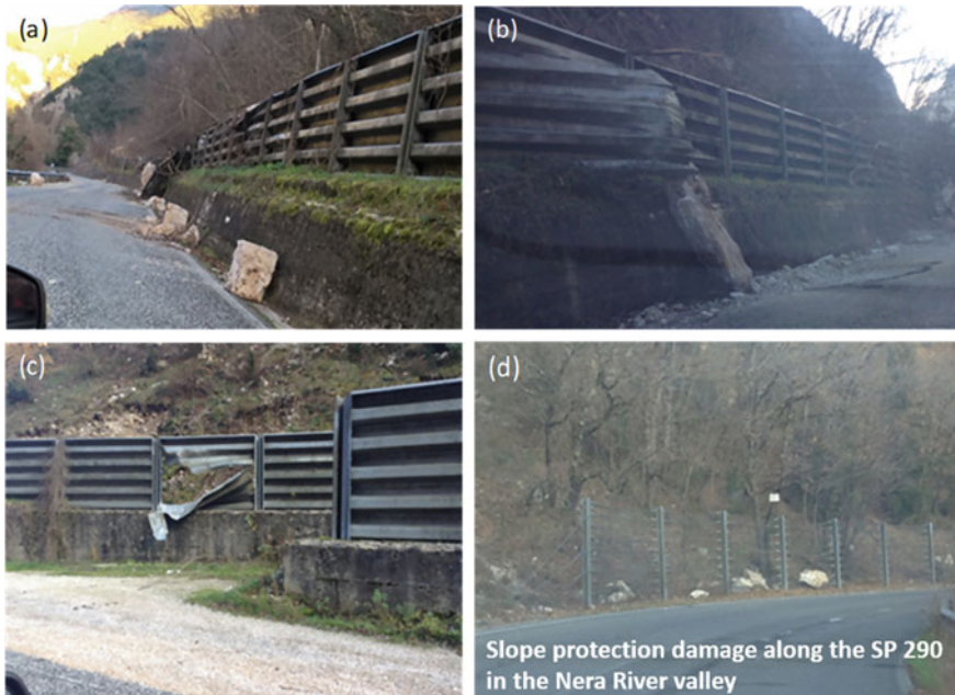
Fig. 25 Slope protection damaged by boulders and rock-blocks along the regional road SP 290 in the Nera River valley (modified from GEER 2017)
