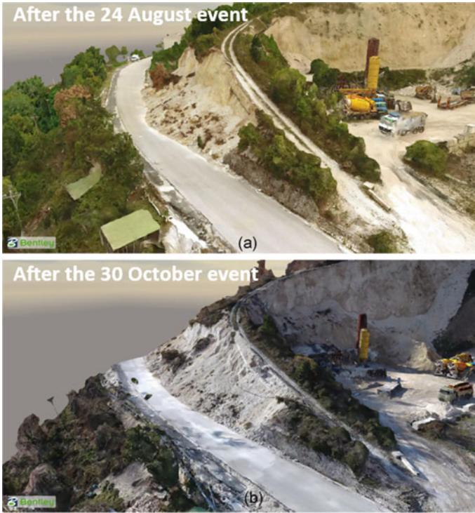
Fig. 34 3D model of landslide #7 and exposed pipeline following: a the 24 August and b the 30 October event (modified from GEER 2017)
