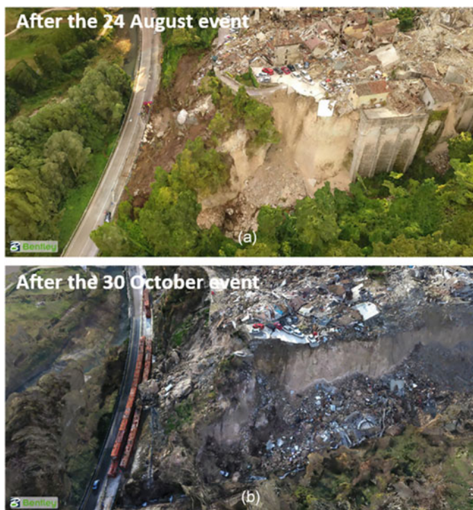
Fig. 31 3D model of the failed retaining wall area in Pescara del Tronto (areas #3–4 in Fig. 28) following: a the 24 August and b the 30 October event (modified from GEER 2017)
