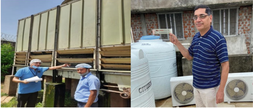
Fig. 3 Reading of operating parameters of cooling tower
