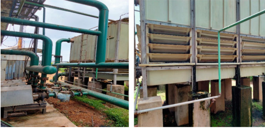
Fig. 2 Induced draft counter flow wet type cooling at VBL, Sanguem, Goa, India
