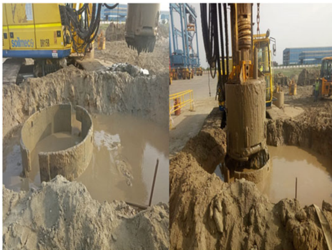
Fig. 23.5 Ponding of drilling mud
