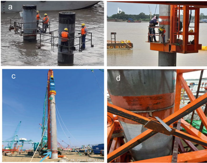
Fig. 29.7 Site photographs of a site setup for cutting of pile segment, b site setup for welding of pile segment, c welded pile segments and d enlarged view of pile welding joint
