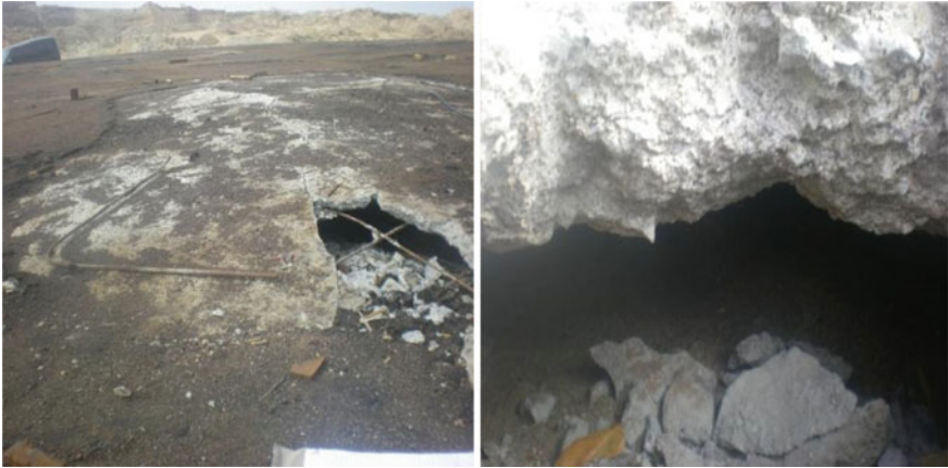
Fig. 28.5 Orientation of failed slab and gap at the central portion of the tank
