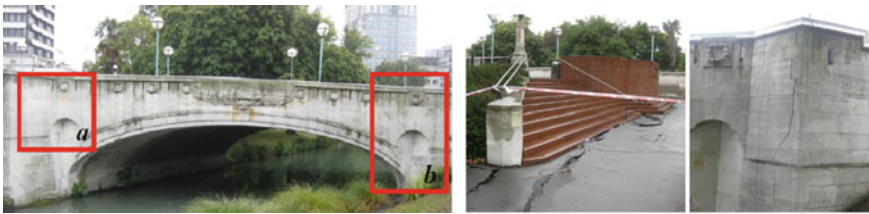
Fig. 13 a Damages to steps on western approach and b Damages to the wingwall on north-eastern wingwall Source (Palermo et al. 2011)
