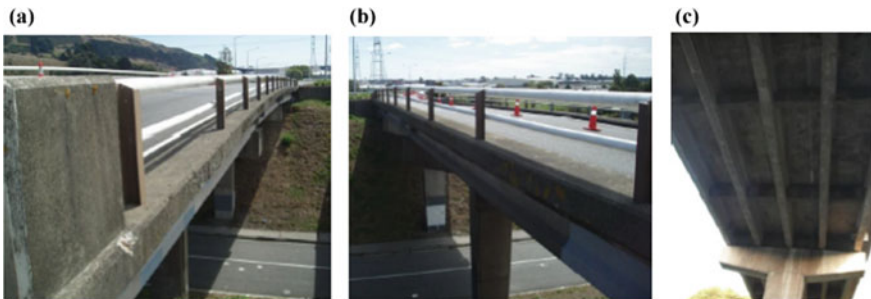
Fig. 18 a-b General view of the superstructure and c deck soffit of the bridge Source (Palermo et al. 2012)
