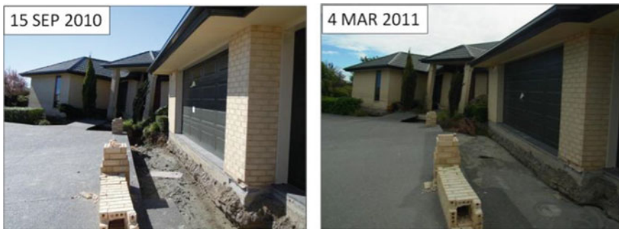
Fig. 9 Damages to residential houses as a result of lateral spreading causing foundation failure during the 2010 Darfield and 2011 Christchurch Earthquake (South Kaiapoi) Source (Yamada et al. 2011)
