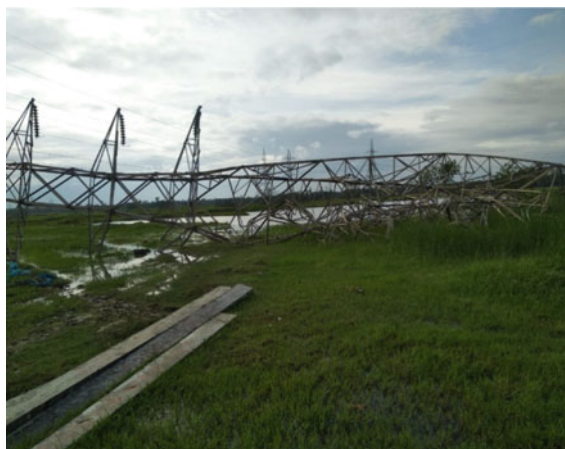
Fig. 6 Completely damaged Transmission Tower due to failure connection with Foundation
