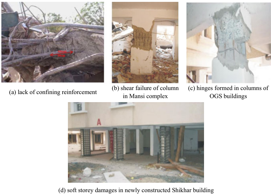
Fig. 3 Identification of damages occurring in RC buildings in Ahmedabad city (Humar et al. 2001)
