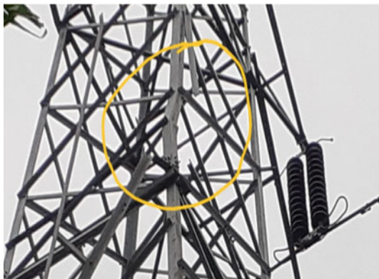
Fig. 5 Partially damaged leg of Transmission Tower
