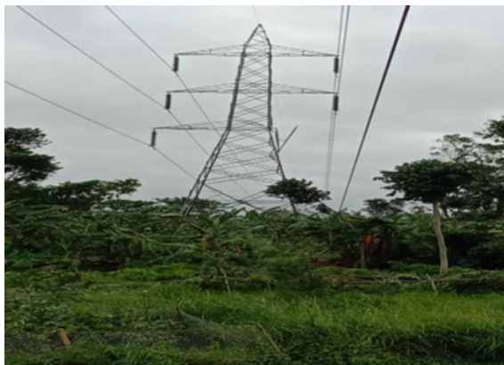
Fig. 4 Partially damaged Cross Arm of Transmission Tower
