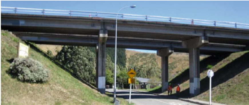
Fig. 17 Overall side view of the Horotane Valley Overpass Source (Palermo et al. 2012)
