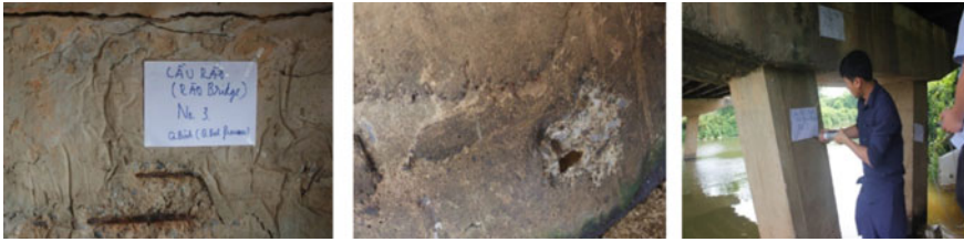
Fig. 2 Damaged images at Rao and Duc Nghia bridges in Quang Binh Province
