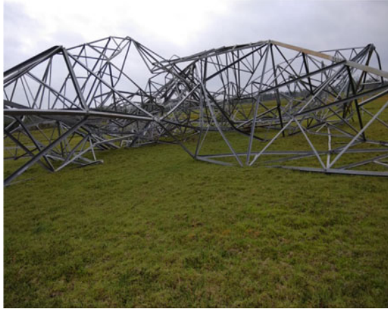
Fig. 7 Completely Damaged Transmission Tower due the Torsional Effect
