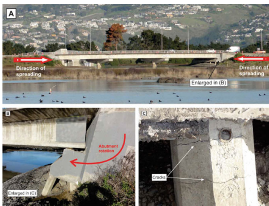
Fig. 4 Typical spreading induced damage to bridges (South Brighton Bridge): A Lateral ground displacement is resisted by the upper bridge structure. B Abutment back-rotation due to the pinning effect and lateral displacement of foundation soils. C Spreading-induced damage (bending cracks) at the top of abutment piles Source (Cubrinovski et al. 2012b)
