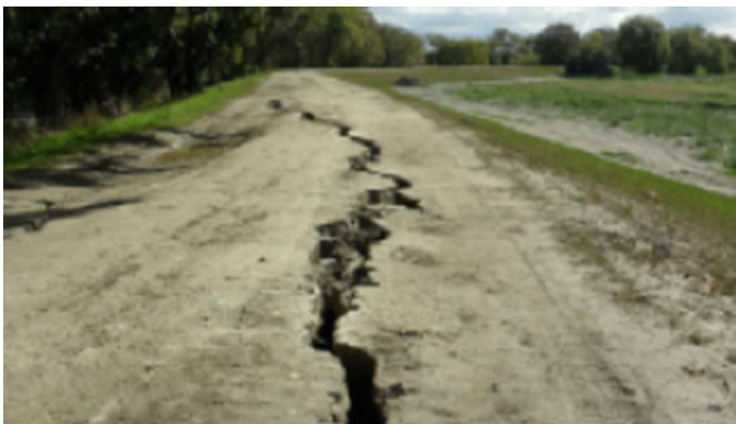
Fig. 11 Example of the longitudinal crack running along the crest of the levee Source (Cubrinovski et al. 2012a)
