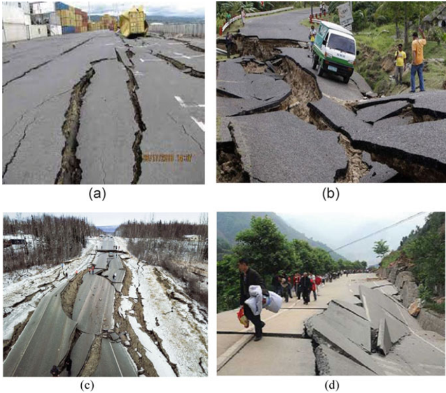
Fig. 1 Road damages due to past earthquakes a Chile earthquake, 2010 b Negros earthquake, 2012(UNDRR, 2012) c Alaska earthquake, 2018 (Structural Engineers Association of Alaska, 2018) d Sichuan earthquake, 2008 (Anbazhagan et al. 2012)
