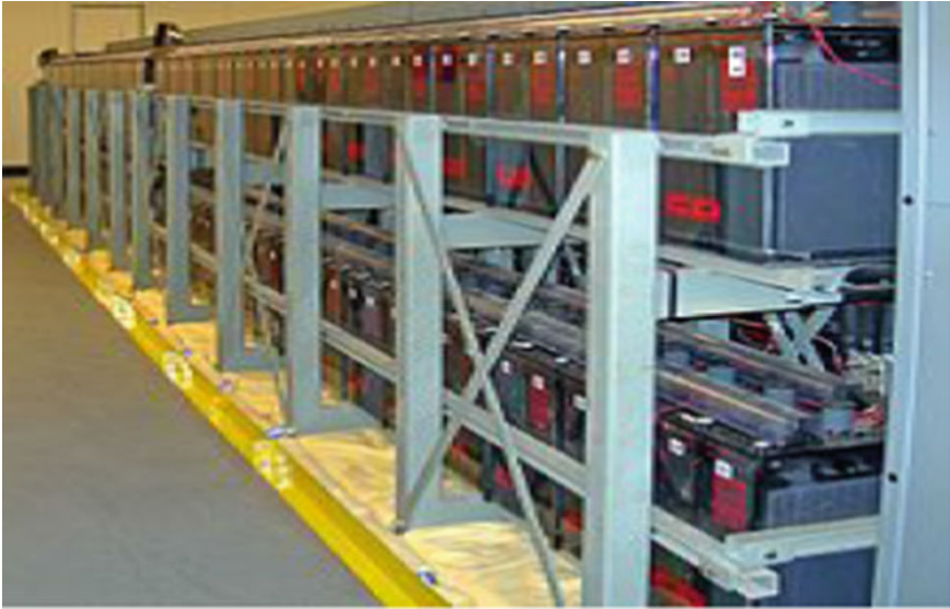
Fig. 3 A bank of batteries in a large data centre used to provide power until diesel generators can start [7]
