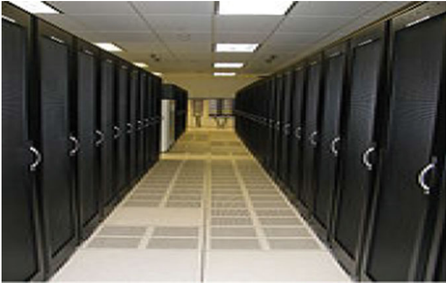
Fig. 4 Typical cold aisle configuration with server rack fronts facing each other and cold air distributed through the raised floor [8]
