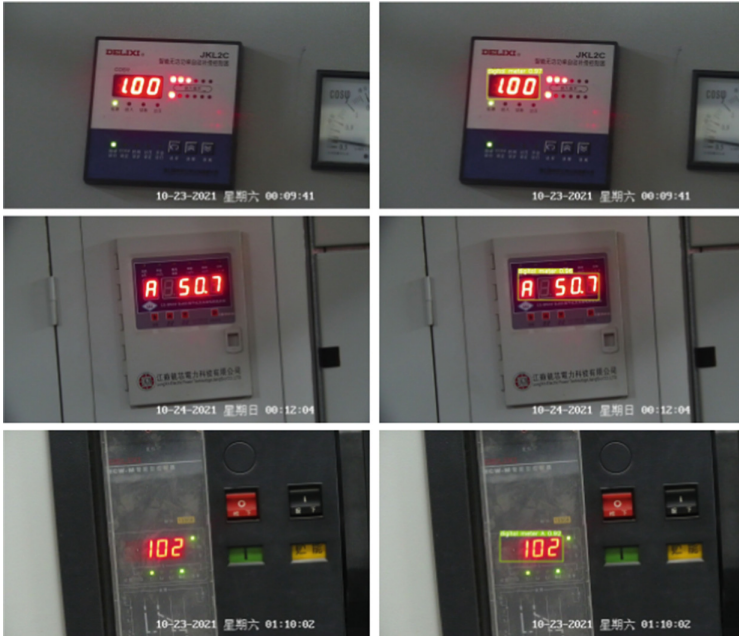
Fig. 9. Distribution cabinet instrumentation character area detection effect
