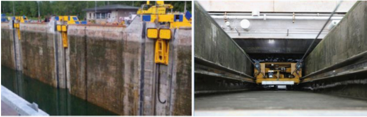
Fig. 11. The vacuum-type automatic floating mooring system
