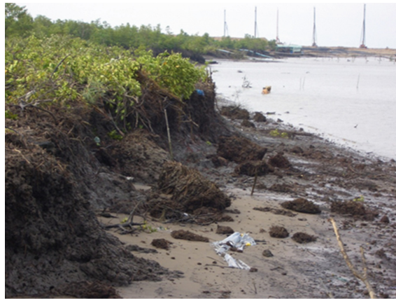
Fig. 3. Condition of river bank
