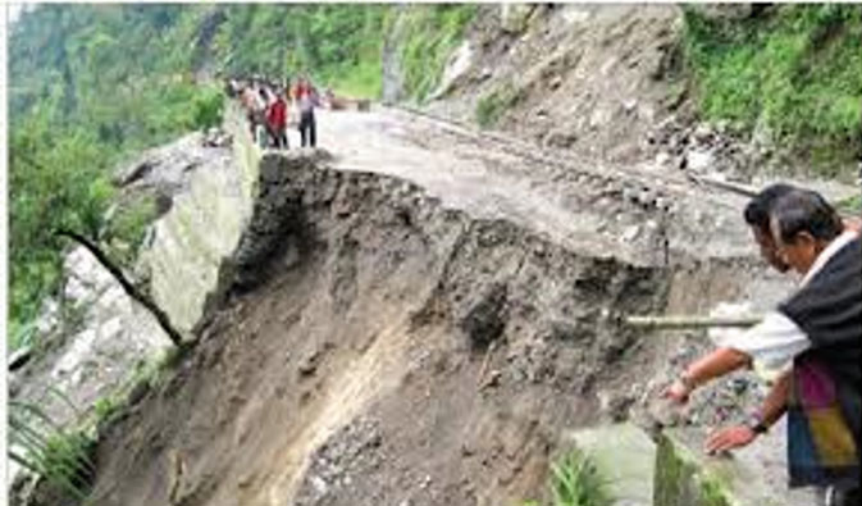
Fig. 3 Landslide along with the road. PC: Vartika Singh
