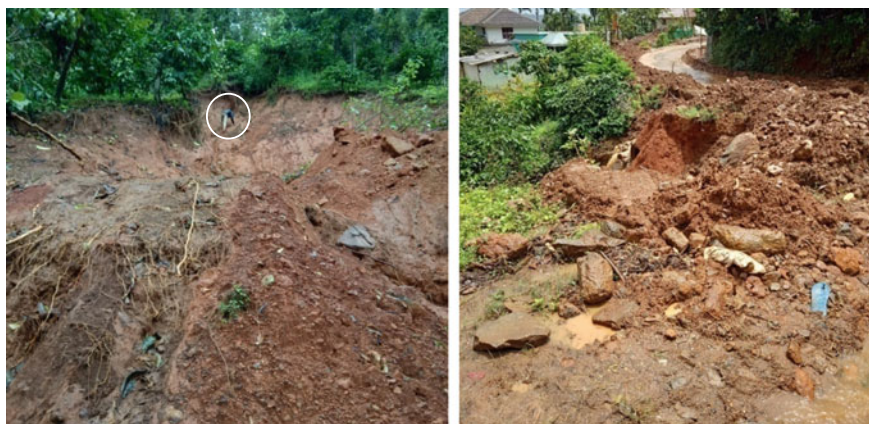
Fig. 8 Two more minor slides that occurred on August 7–8; one of the authors (circled) climbing a slide. Some of the slides occurred along the tributaries of the Pachakkad-Puthumala thodu [12]
