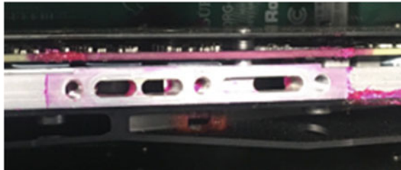
Fig. 39 Coolant leakage in waterblock/manifold (pink color)
