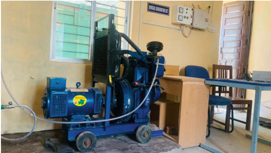
Fig. 2 Biogas generator set (dual fuel-based- diesel and biogas)
