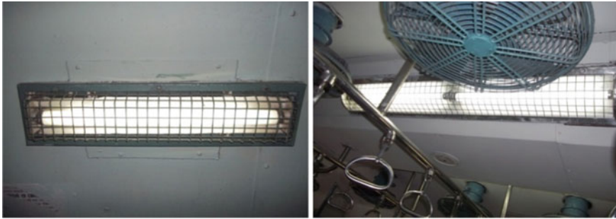
Fig. 1 Lighting fixture of old and new EMU coach
