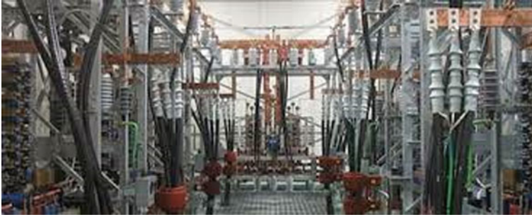
Fig. 1 Showing an installed SVC in Kanpur 400 kV substation
