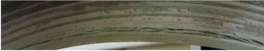
Fig. 2 Delaminated FRP ring 1
