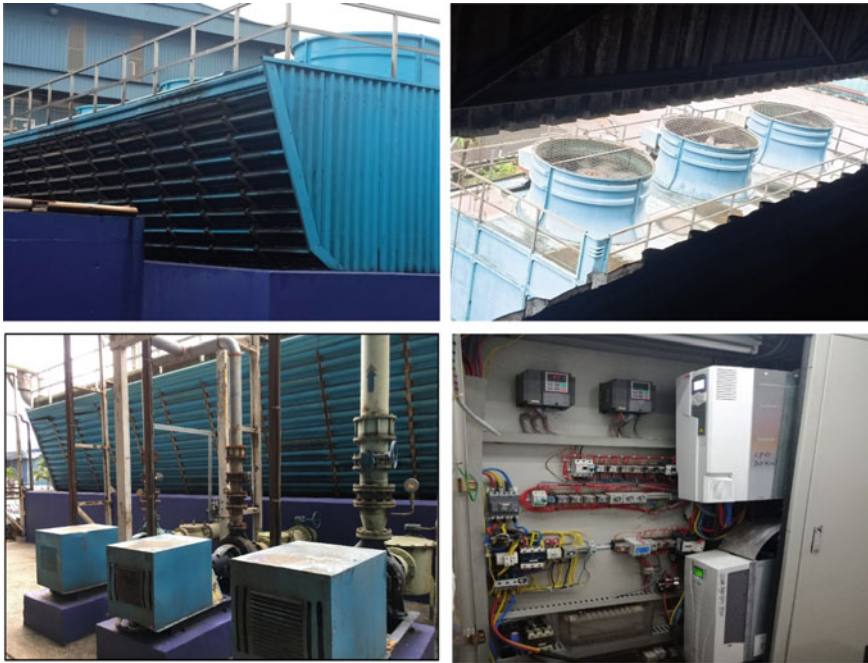
Fig. 8 Usage of inverter for cooling tower fans and pumps
