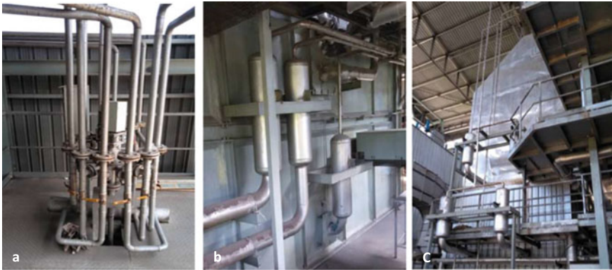
Fig. 14 Shock wave soot blasters a Distributor header, b Mixing chamber and inlet nozzles (silver colored) placed horizontally, and c Mixing chamber and inlet nozzles placed around the economizers
