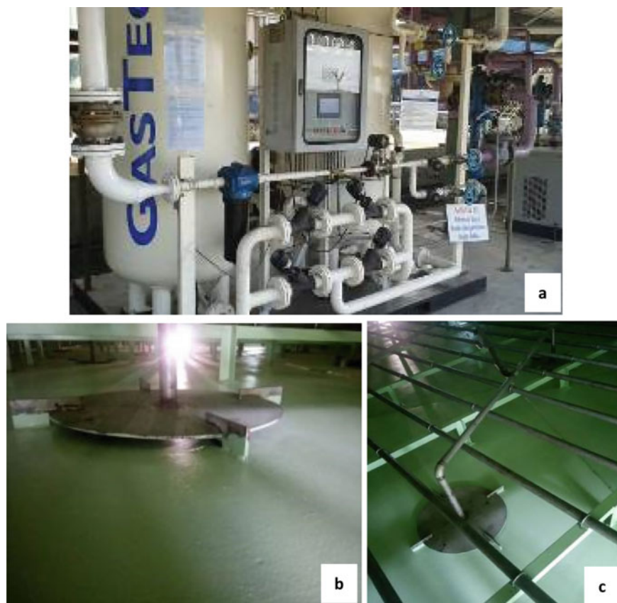
Fig. 17 a PSA nitrogen generation plant; b, c Nitrogen is pulse-bubbled into storage tanks to preserve the quality of its contents
