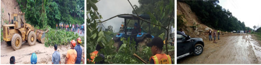
Fig. 25 Landslide on nearby roads being cleared by IOIEO personnel and equipment
