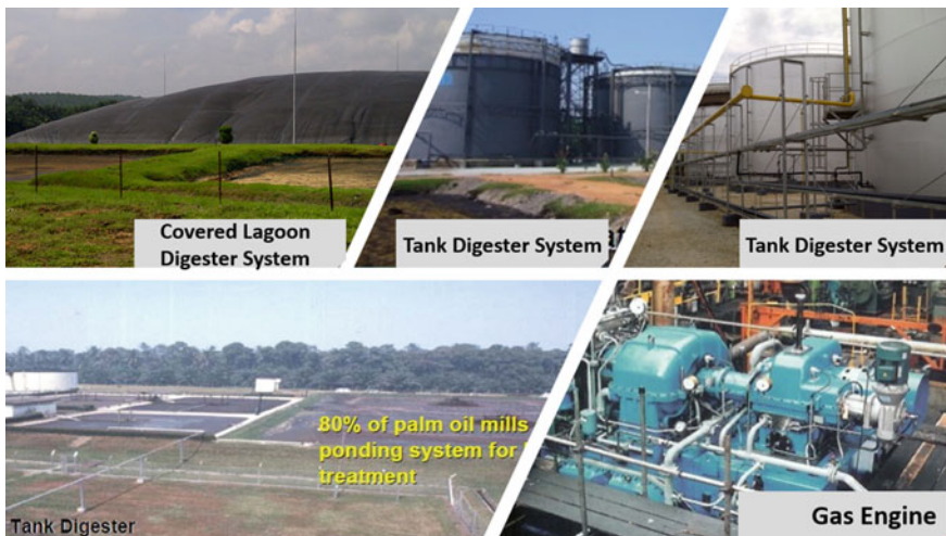
Fig. 26 A biogas system—tank digester system, covered lagoon digester system, and a gas engine
