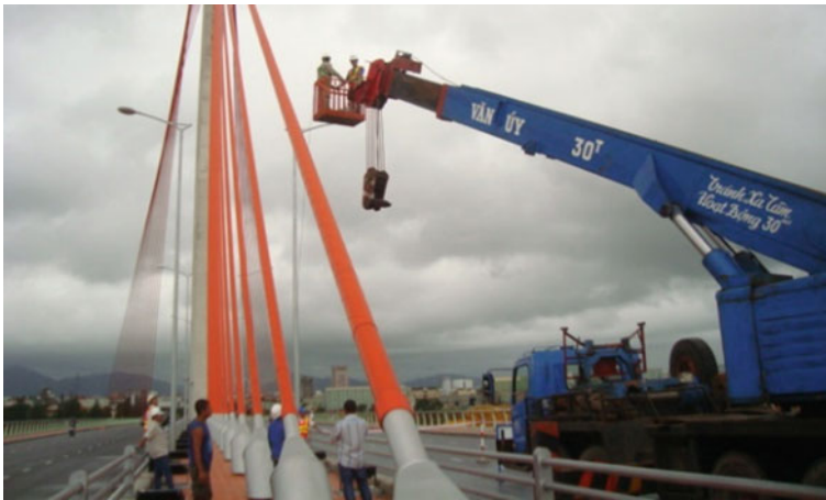
Fig. 3 Installation of the accelerometers for damping test on the Tran Thi Ly stay cable bridge (photo provided by VSL Vietnam)
