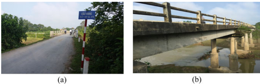
Fig. 2 Vang bridge: a the top view of the bridge; b downstream side of the bridge
