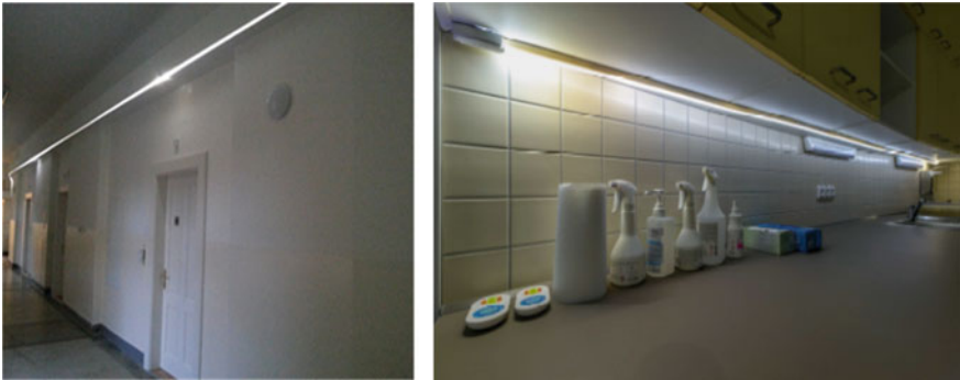
Fig. 5.35 Emergency lighting in hospital
