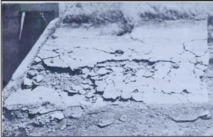
Fig. 2 Disintegration of concrete due to sulfate attack [5]
