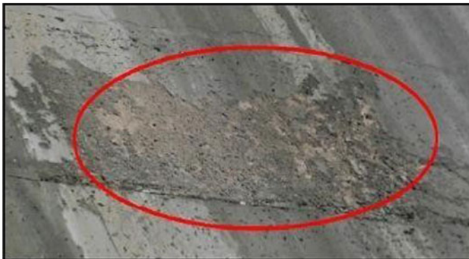
Fig. 1 Disintegration of concrete surface at dam face [5]
