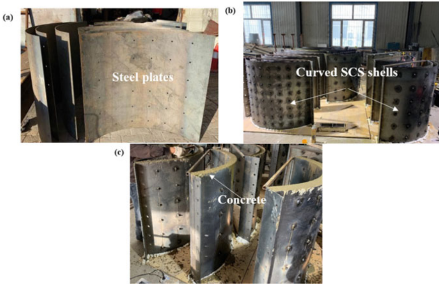
Fig. 7.2 Fabrication process: a rolling steel plates into curved shape, b erecting CSCS sandwich shells and c casting concrete, reprinted from Yan et al. (2020a), copyright 2022, with permission from Elsevier
