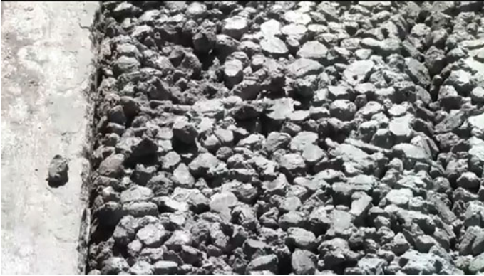
Fig. 2 Raveling in pavement
