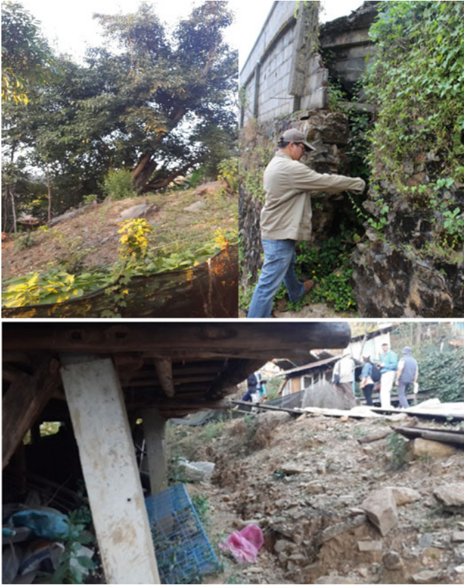
Fig. 5.4 Observed movement of house and infrastructure in Doi Chang village, Chaing Rai, Thailand
