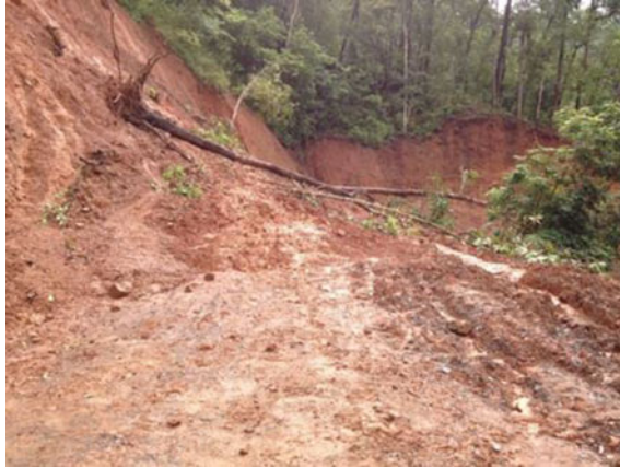
Fig. 5.2 Slope failure in cut slope
