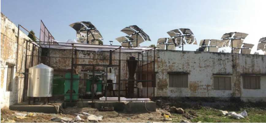
Fig. 3 Site photograph of solar thermal system
