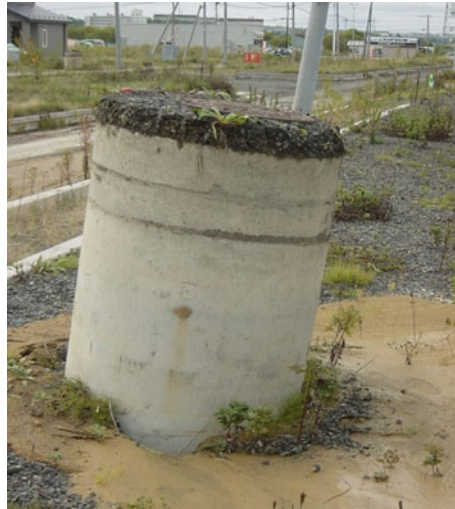
Fig. 4 Upliftment of Manhole due earthquake-induced liquefaction
