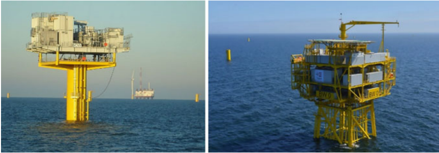
Fig. 16 Photographs of offshore substations. Source http://www.trianel-borkum.de/en/kraftwerk/converter-platform/ and https://commons.wikimedia.org/wiki/File:Offshore-132kv-Substation.jpg
