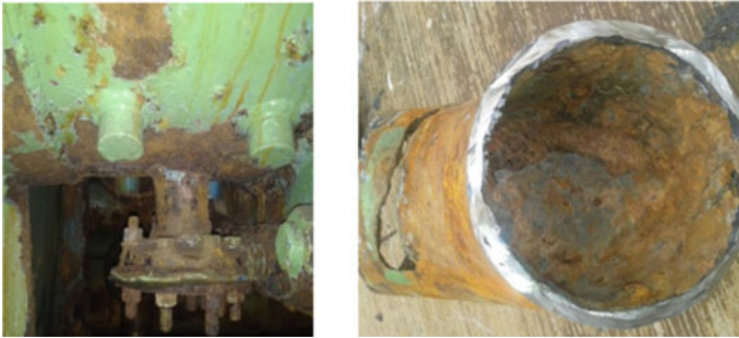
Fig. 5 Cooling water pipe corrosion at power plant
