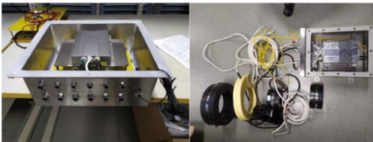
Fig. 7 High-voltage grounding current monitoring system of the cable
